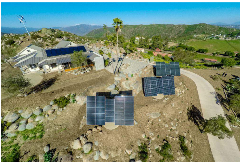
Casa Aguila's solar trackers. (Photo credit: KNB Associates, LLC.)
