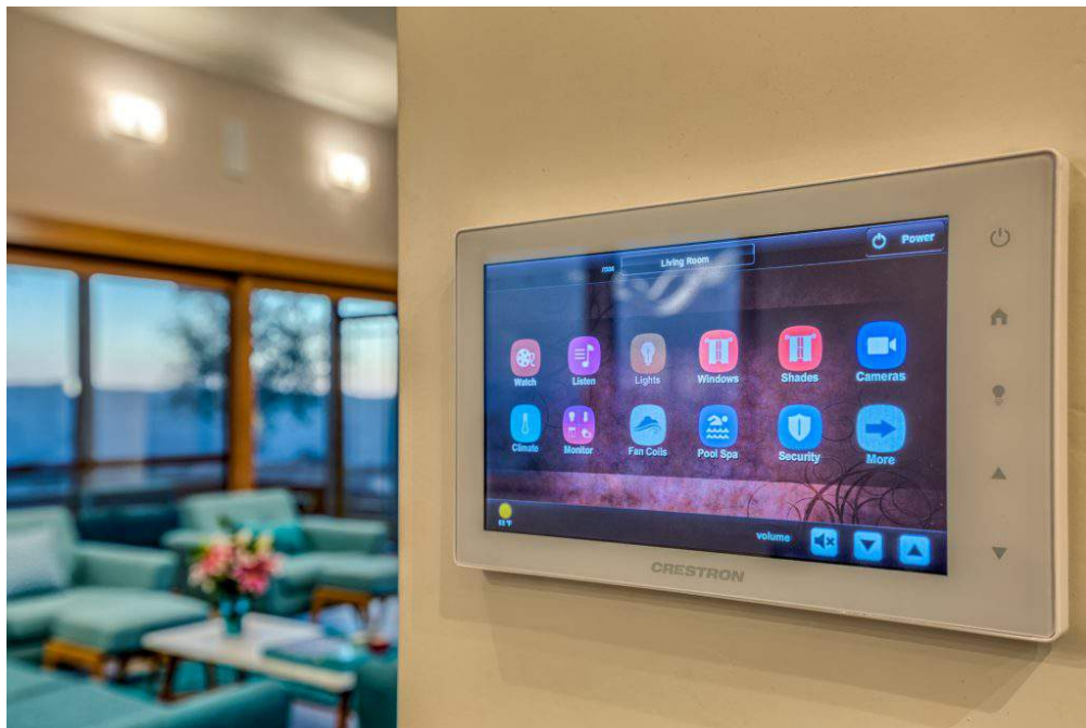
Casa Aguila's Crestron System. (Photo credit: KNB Associates, LLC.)
